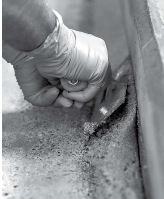
Above: A cove base installation showcases the seamless, hygienic design of Sherwin-Williams flooring systems, built for the rigorous demands of food and beverage processing facilities.
